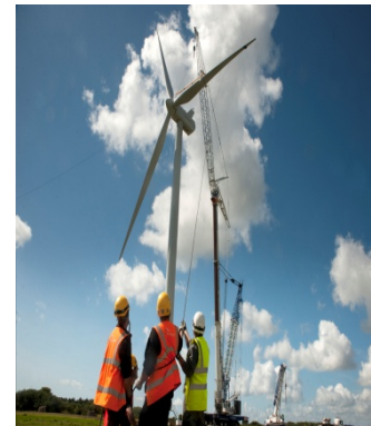
Goonhilly Downs Wind Farm
