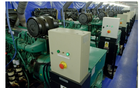
REG Bio-Power's Bentwaters plant operates 6MW of our STOR contract
