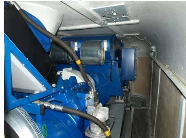
Inside of AW1500 Nacelle.
